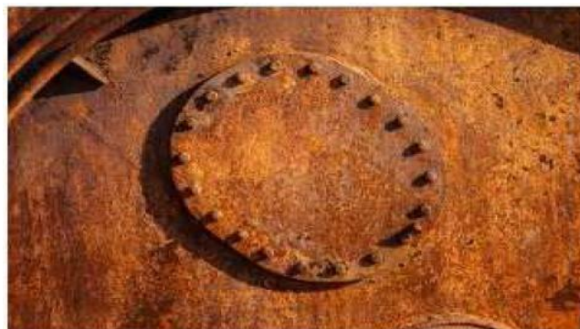
Fig.1 General Corrosion on Mechanical Parts
