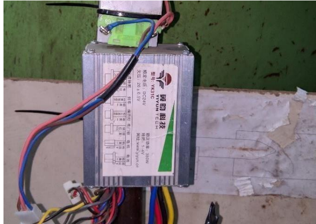
Fig. 6. PWM motor controller as installed.
